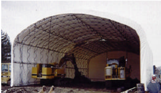
Two MITU-12 Units Beneath Structure Arcade, NY
